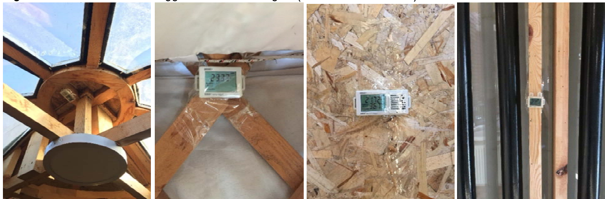
Figure 3B. Data loggers installed into the Ger Plug-in
